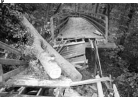
Sections of the Saunders-Monticello Trail boardwalk were destroyed in the storm.
