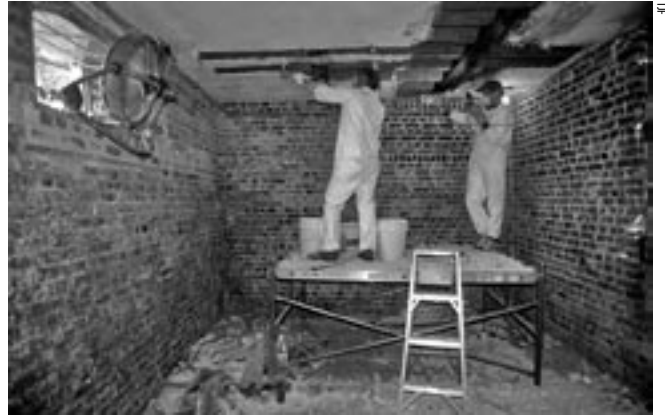
Monticello's Bob Self (left) and Rob Newcomb removing the Wine Cellar's mid-20th century plaster ceiling.
