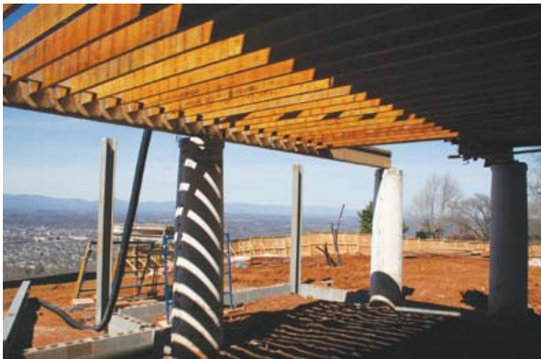
Repose, the house atop Montalto that dates to the early 1900s, is being restored and renovated to accommodate a wide range of programs and events. T.J.F.
